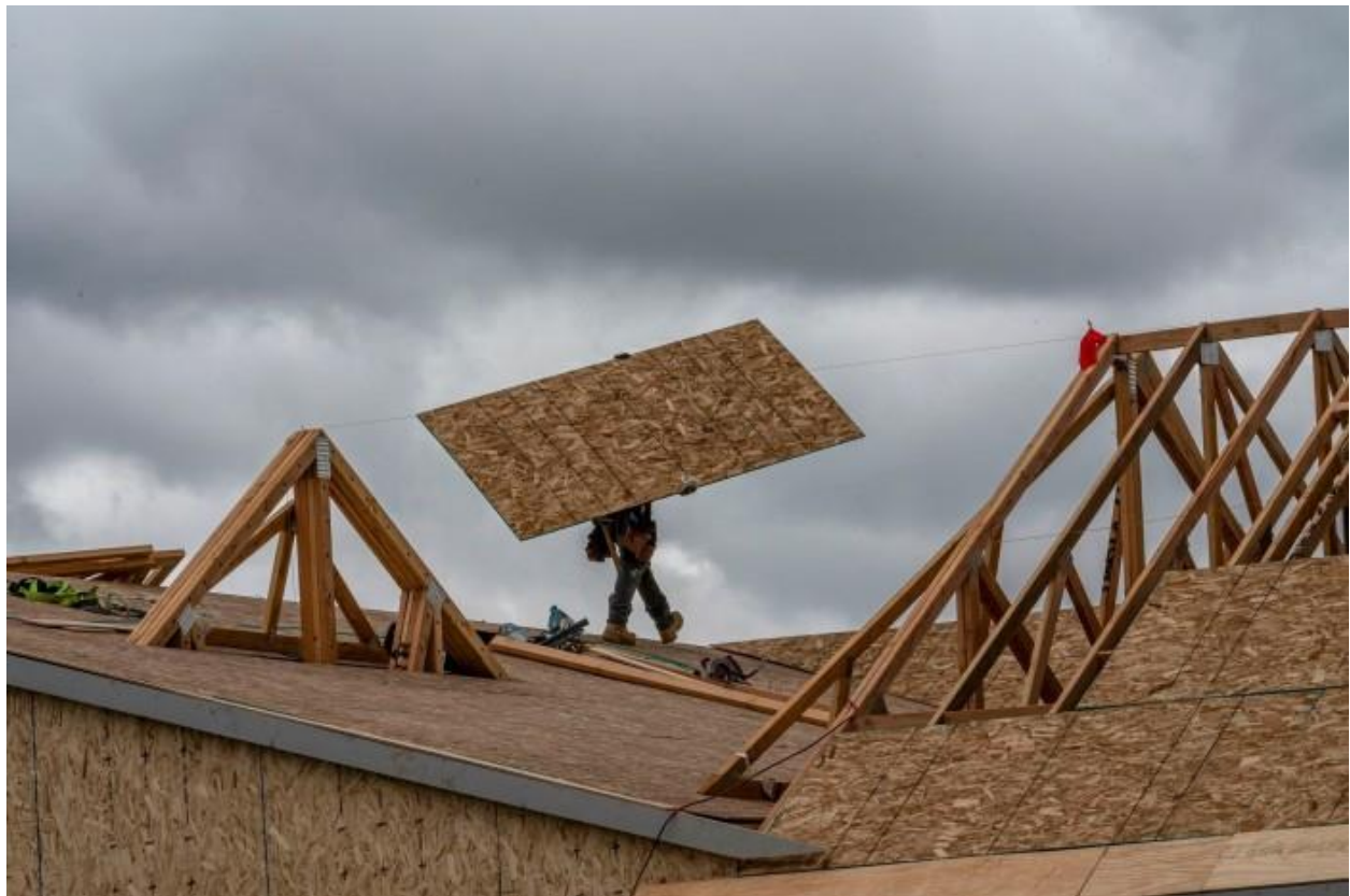
A contractor on the roof of a home under construction. DAVID PAUL MORRIS/BLOOMBERG NEWS
