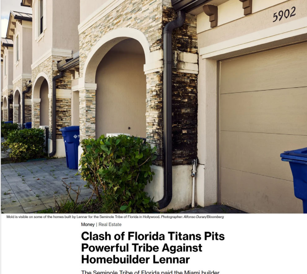
Mold is visible on some of the homes built by Lennar for the Seminole Tribe of Florida in Hollywood. Photographer: Alfonso Duray/Bloomberg
